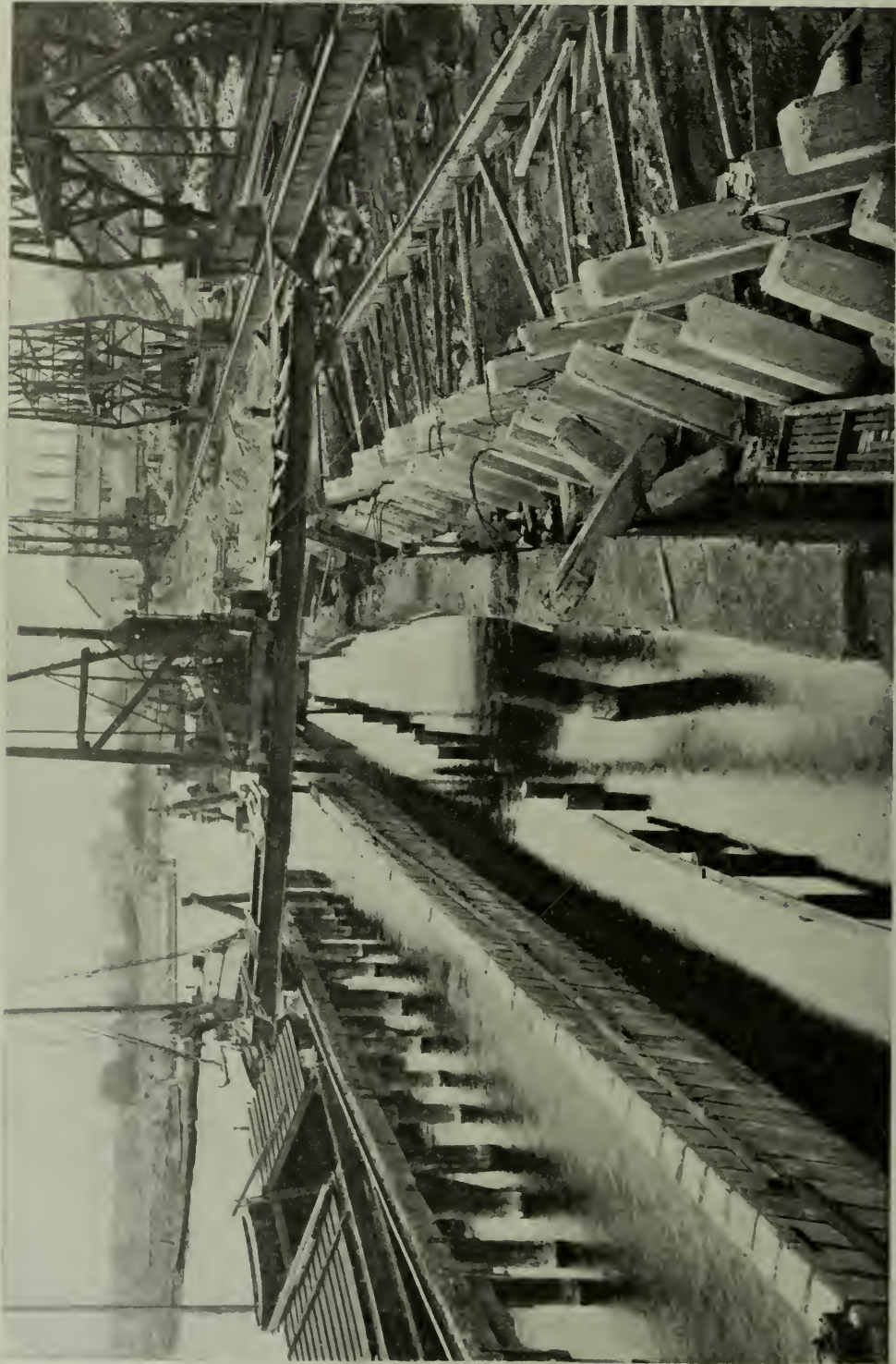
FIG. 10.—SUBSTRUCTURE FOR QUAY WALL CONSISTING OF FRONT SHEET PILES AND BACK YOKE PILES.
